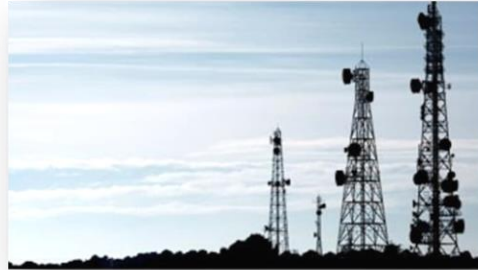
Ground Based Tower
