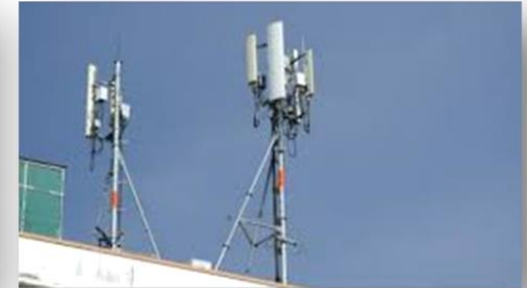
Roof Top Tower
