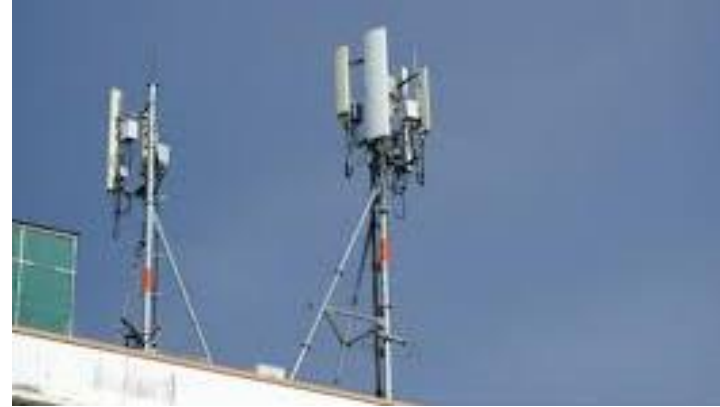
ROOF TOP TOWER
