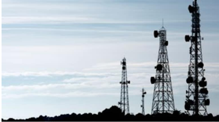
GROUND BASED TOWER
